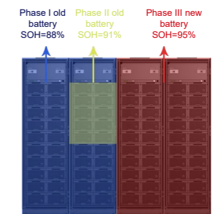
More flexible mixing of old and new batteries
